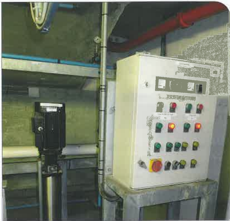
High pressure pump and control panel.
